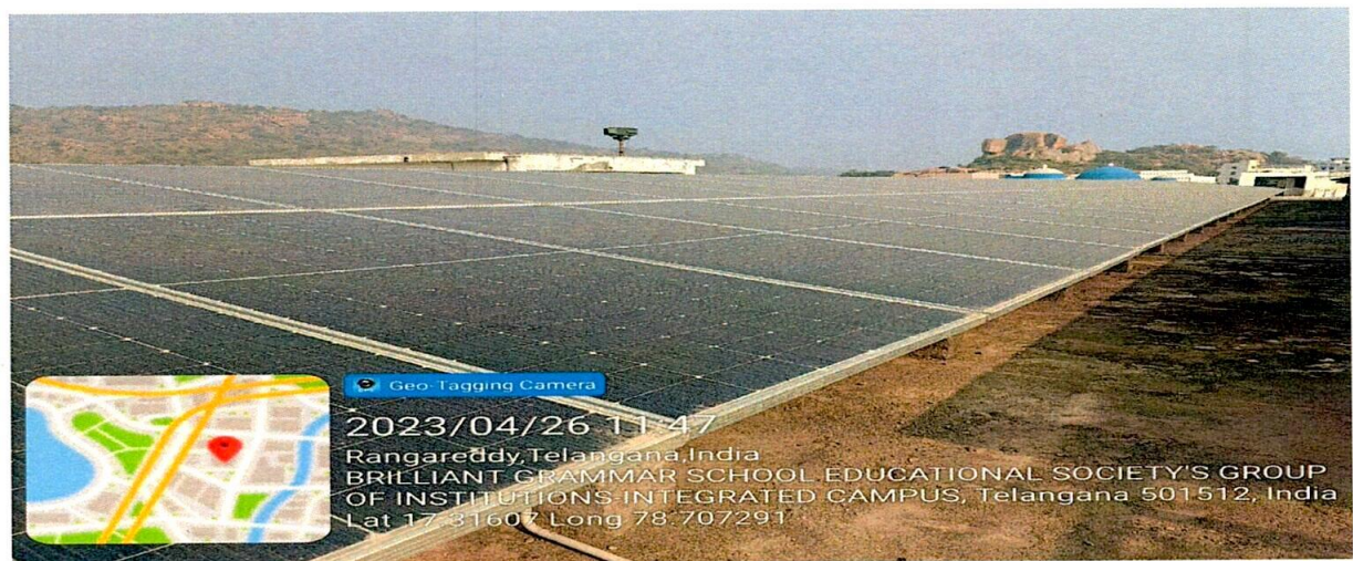
View of Solar Power plant 75 KWp.
