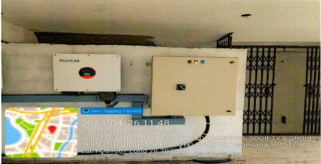
Wheeling to GRID connection.
